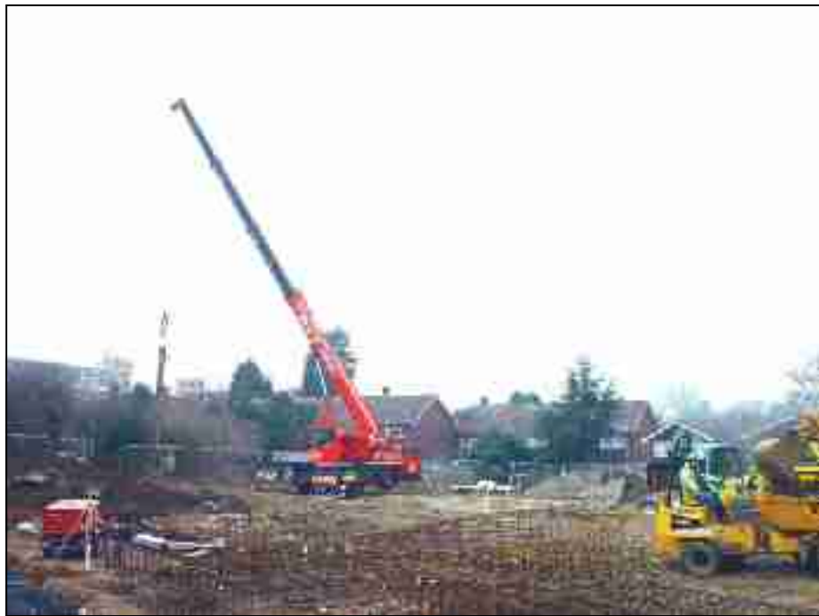
The building site in the process of being converted into houses and the new Doctor's Surgery—photo by James Millham
